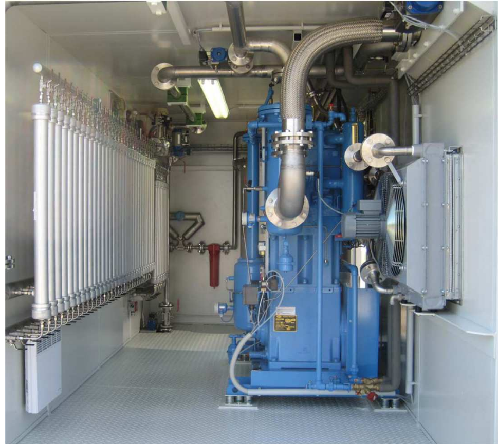
Impianto a membrane in container – Bruck an der Leitha - Austria
